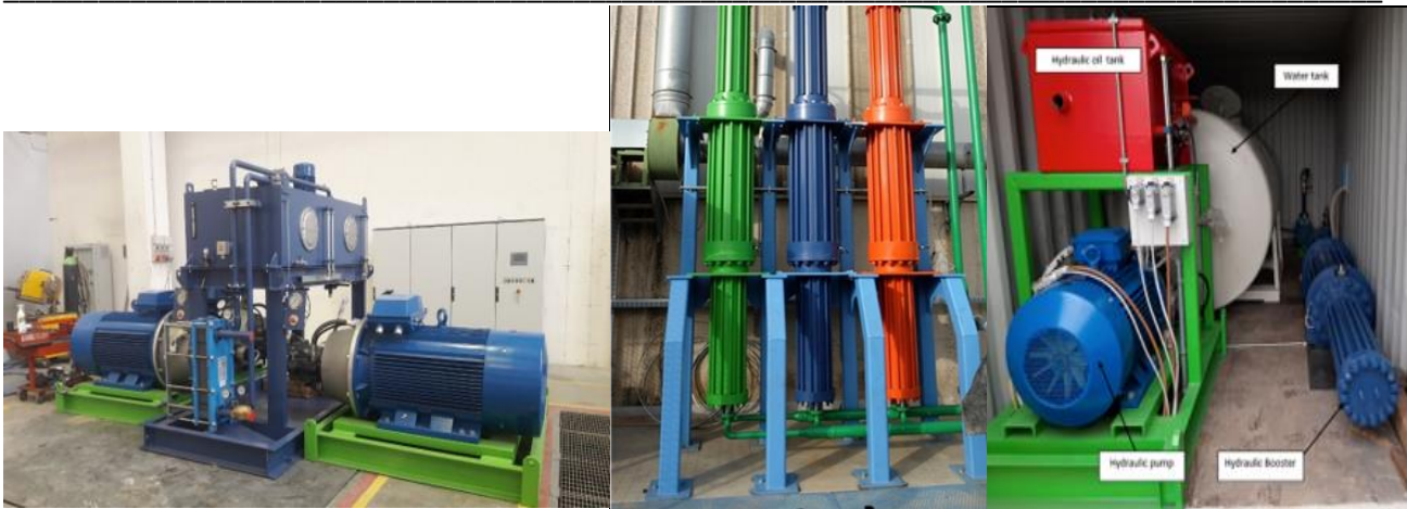
PUMPING UNIT FOR AUTOFRETTAGE AND 10000 CYCLES FATIGUE
